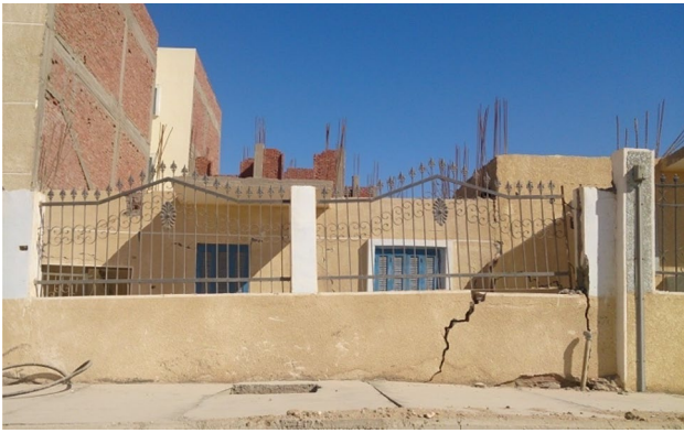
Fig. 6 Current structure problems of some Ibny Baitak buildings in NAC (pictured in July 2023) [1]
