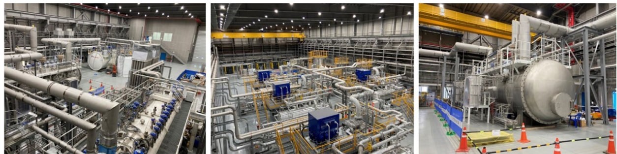
Fig. 6 Images of the cryoplant system. From left to right, a cold box, warm compressors, and the liquid-He distribution system along with a cold box are shown
