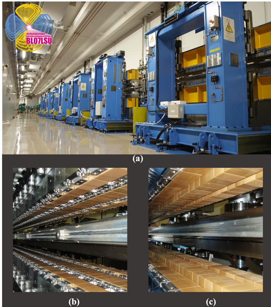
Fig. 1 Photos of the first segmented cross undulator, "ID07," installed at the University-of-Tokyo Outstation Beamline for Materials Science, SPring-8 BL07LSU [27]. a A set of the eight ID segments of undulators. b,c Arrays of magnets in b the horizontal figure-8 undulator segment and c the vertical figure-8 undulator segment
