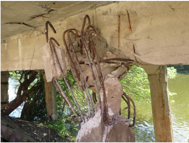
Fig. 13 View of the damaged RC wharf structure
