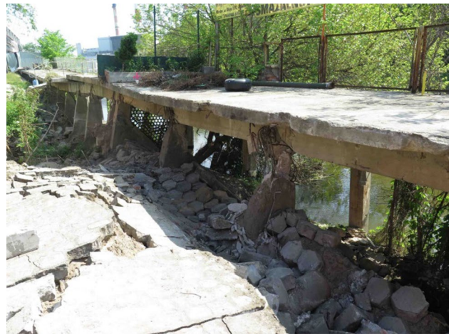
Fig. 11 View of the embankment part of the damaged RC wharf
