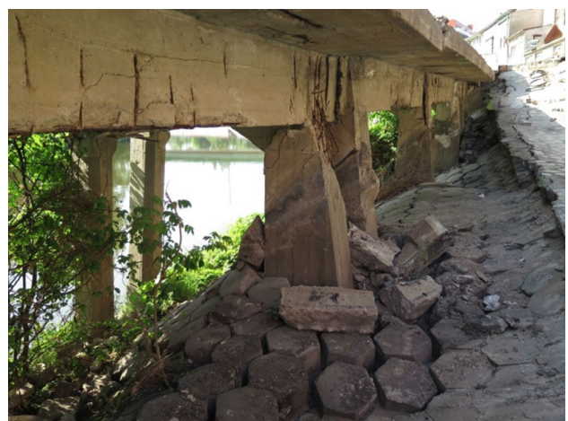
Fig. 12 View of the damaged RC wharf structure
