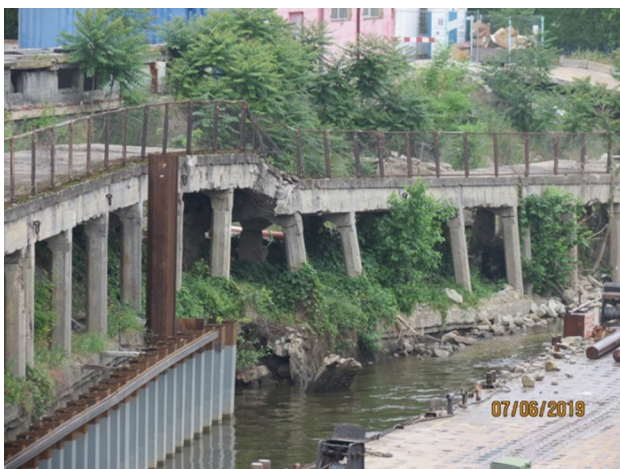
Fig. 10 General view of the destroyed RC wharf
