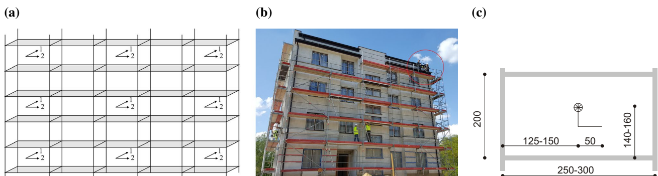
Fig. 1 Location of measurement points on the scaffolding: a diagram of sample locations and directions of wind speed axes, b measurements performed on site, and c front view of the measurement layout on a single level for a perpendicular component of wind speed (axis 1)
