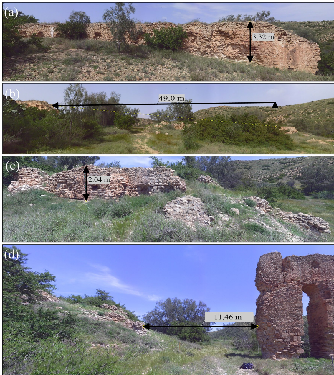
Fig. 5 View from west to sections A (a), B (b), C (c), and D (d) of the CAB 3D scan model
