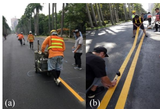
Fig. 7. Field construction of (a) thermoplastic road markings and (b) preformed pavement marking tapes.
