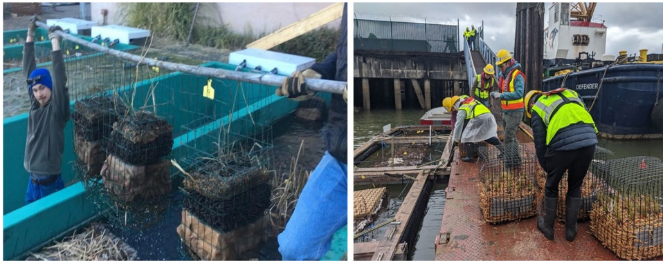
Fig. 4 Construction of prototypes for the Duwamish Floating Wetlands Project. Images show students constructing floating wetland “Biofilters” at an underutilized hatchery in February 2019 (left) and community members and the academic team installing the Biofilters
