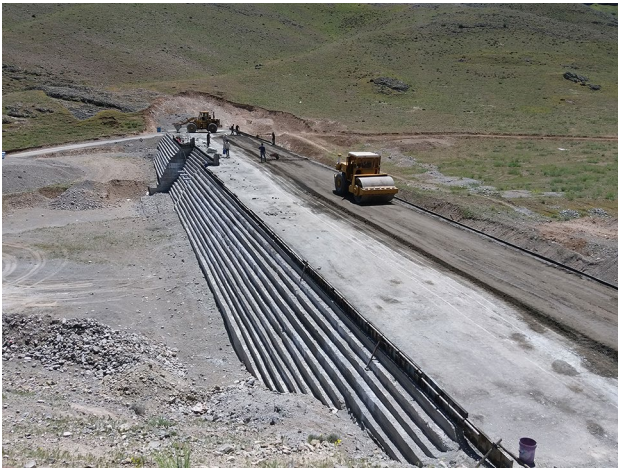
Fig. 2 The CSG check dam in the Marand city of Iran during construction
