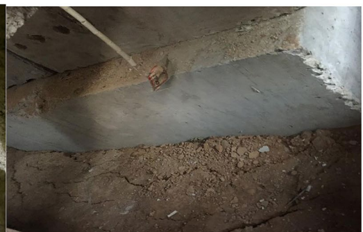
(e) Cracks on the ground surface
