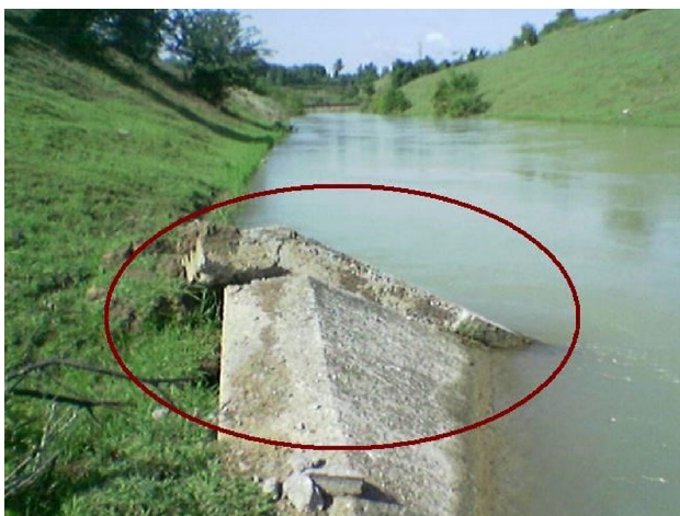
Fig. 2 The slope instability in the right Sangar's canal bank
