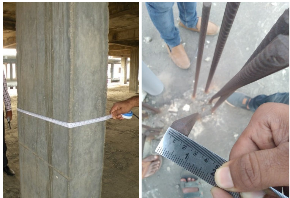
Fig. 5 Verification of dimensions and cross-sectional details of beams and columns during field visits
