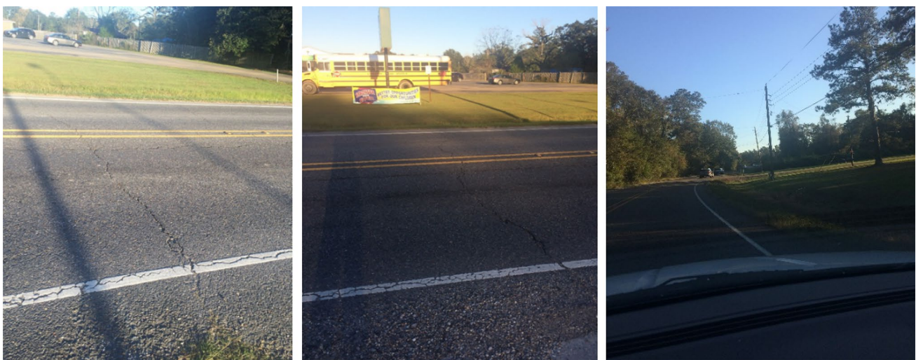
Fig. 9 Existing road conditions of LA 22
