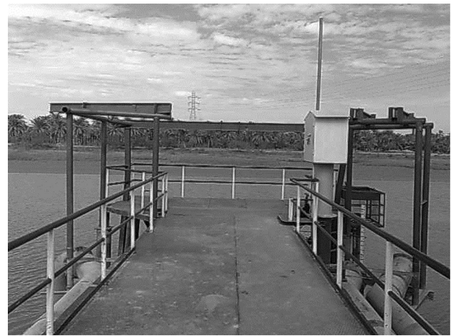
Fig. 3 Suction pipes of the Bavi pumping station
