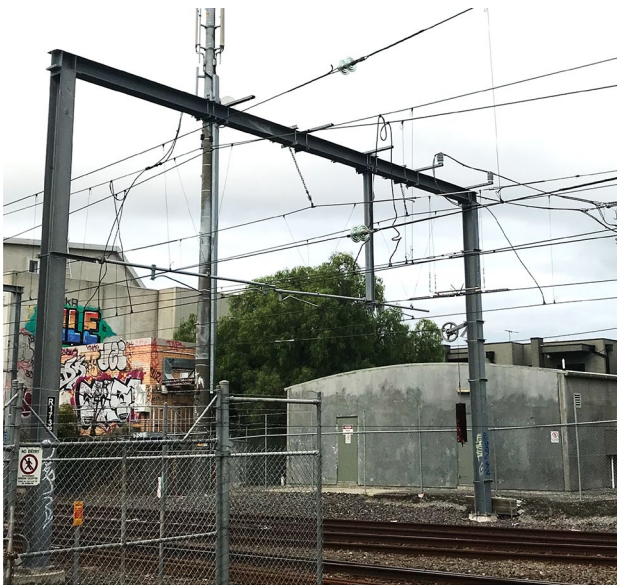
Fig. 1 Portal type overhead wiring structure
