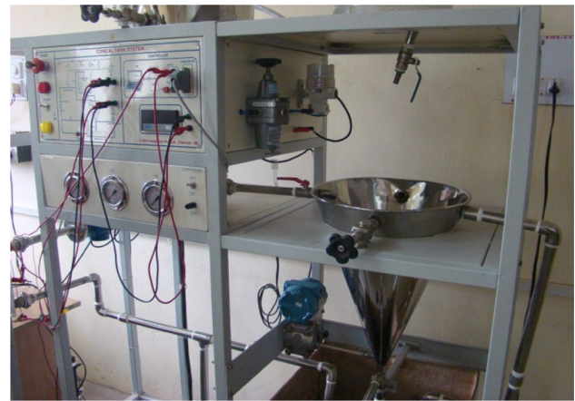
Fig. 3 Real time setup of a single conical tank system
