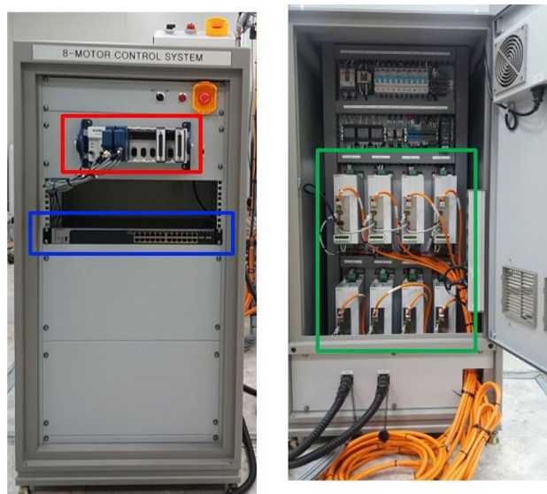
Fig. 7 19-inch rack system integrating the electric hardware
