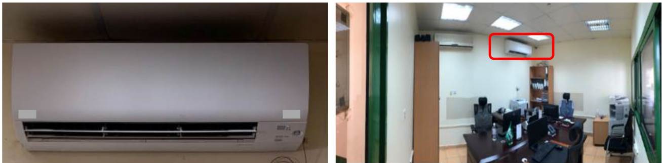
Fig. 2 Room of inverter unit
