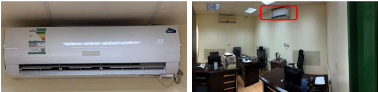
Fig. 3 Room of non-inverter unit
