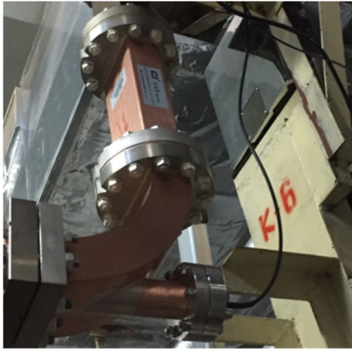
Fig. 4 Installed arcing detection module (top) and E-bend waveguide observation window with optical fiber (bottom)
