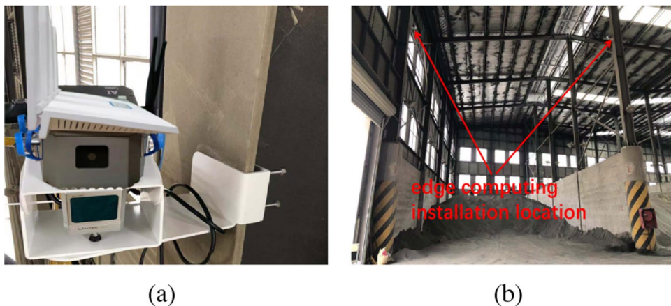
Fig. 3 The module installed on the warehouse
