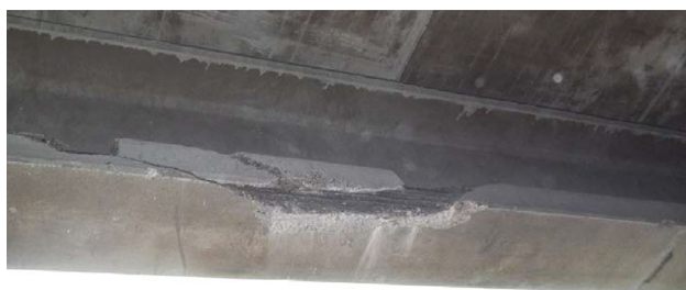
Fig. 3 Damaged girder photograph
