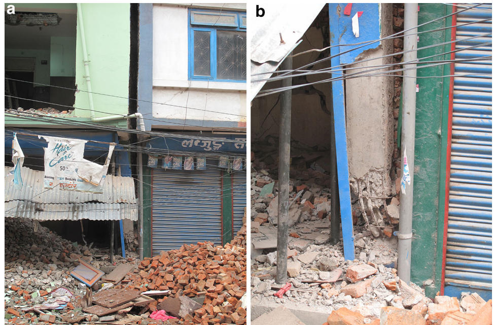
Fig. 1 RC column damaged after the Gorkha 2015 earthquake in Nepal. a General view of the RC column. b Plastic hinge in the base of the RC column
