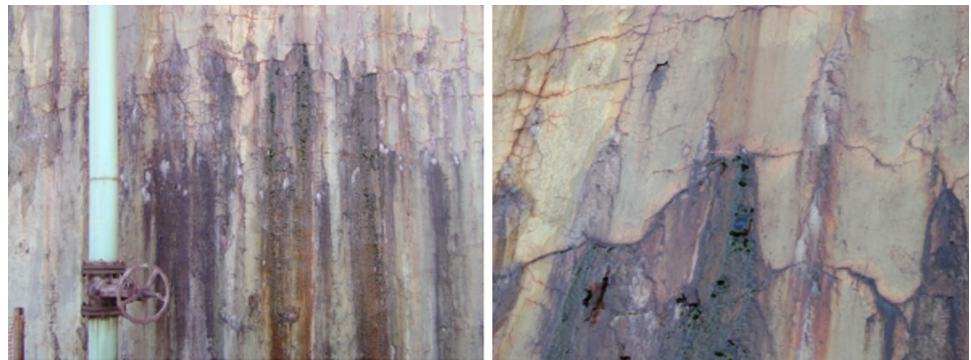
Fig. 4 Details of the reservoir wall presenting fissuration and water percolation
