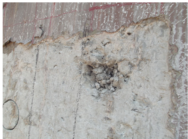
Fig. 5 Segregated concrete point visualized after a partial removal of the coating
