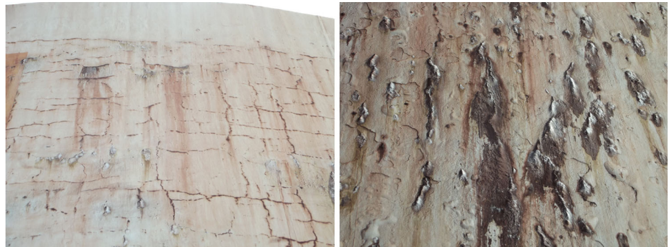
Fig. 2 Fissuration details on the reservoir wall. Note also the presence of failure in water-tightness and deterioration of the coating
