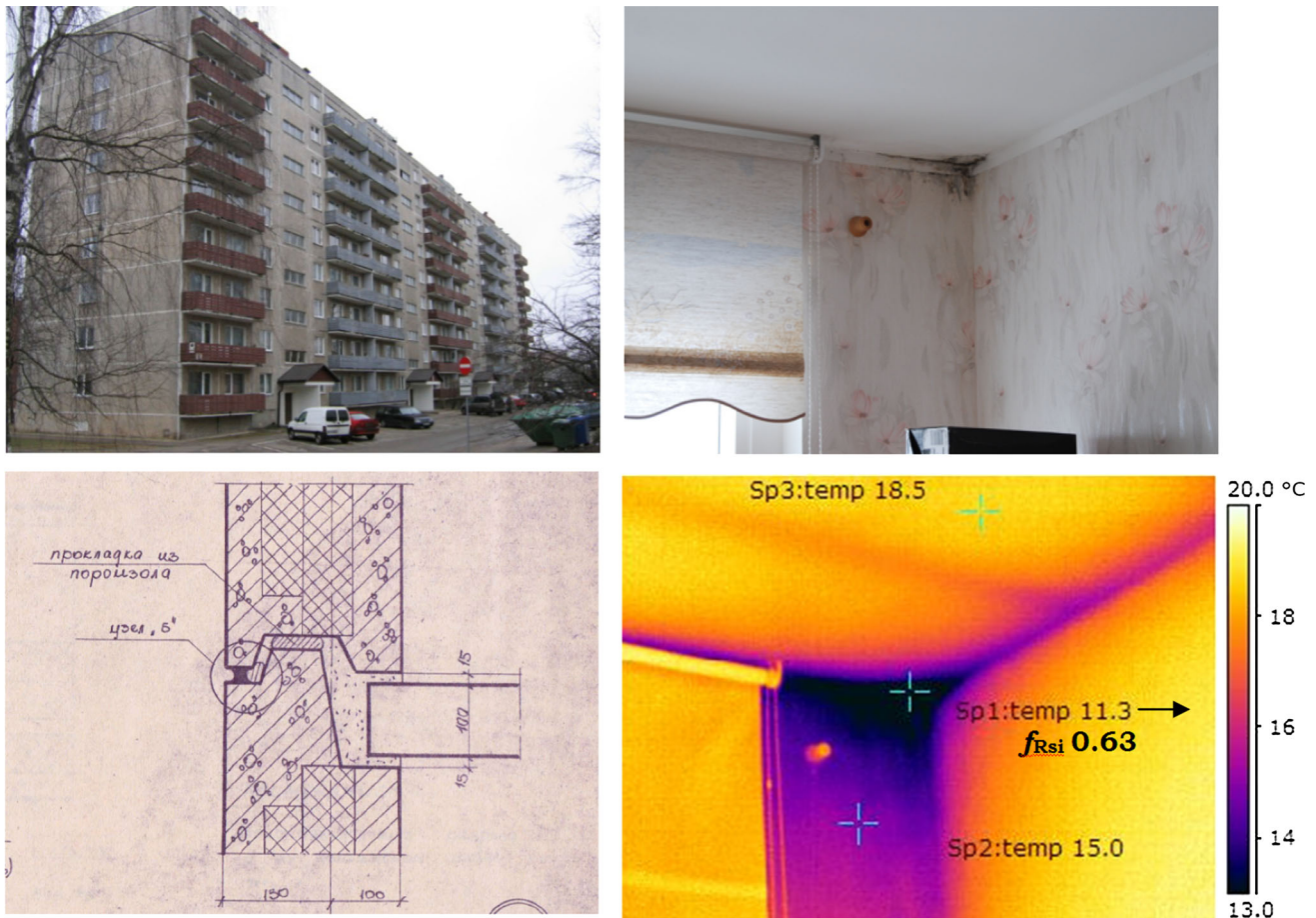
Fig. 4 Example of a precast concrete large-panel apartment building (upper left) with discontinued insulation in the junction of the external wall and floor (lower left). Visible mould growth at the corners of a
