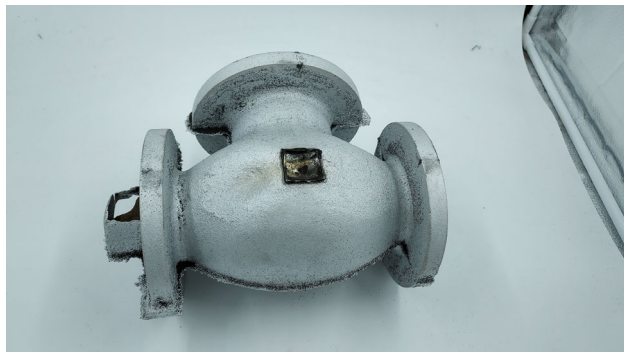
Figure 13. Valve body casting with inadequately filled and vented tag, the same part as Figure 12c.
