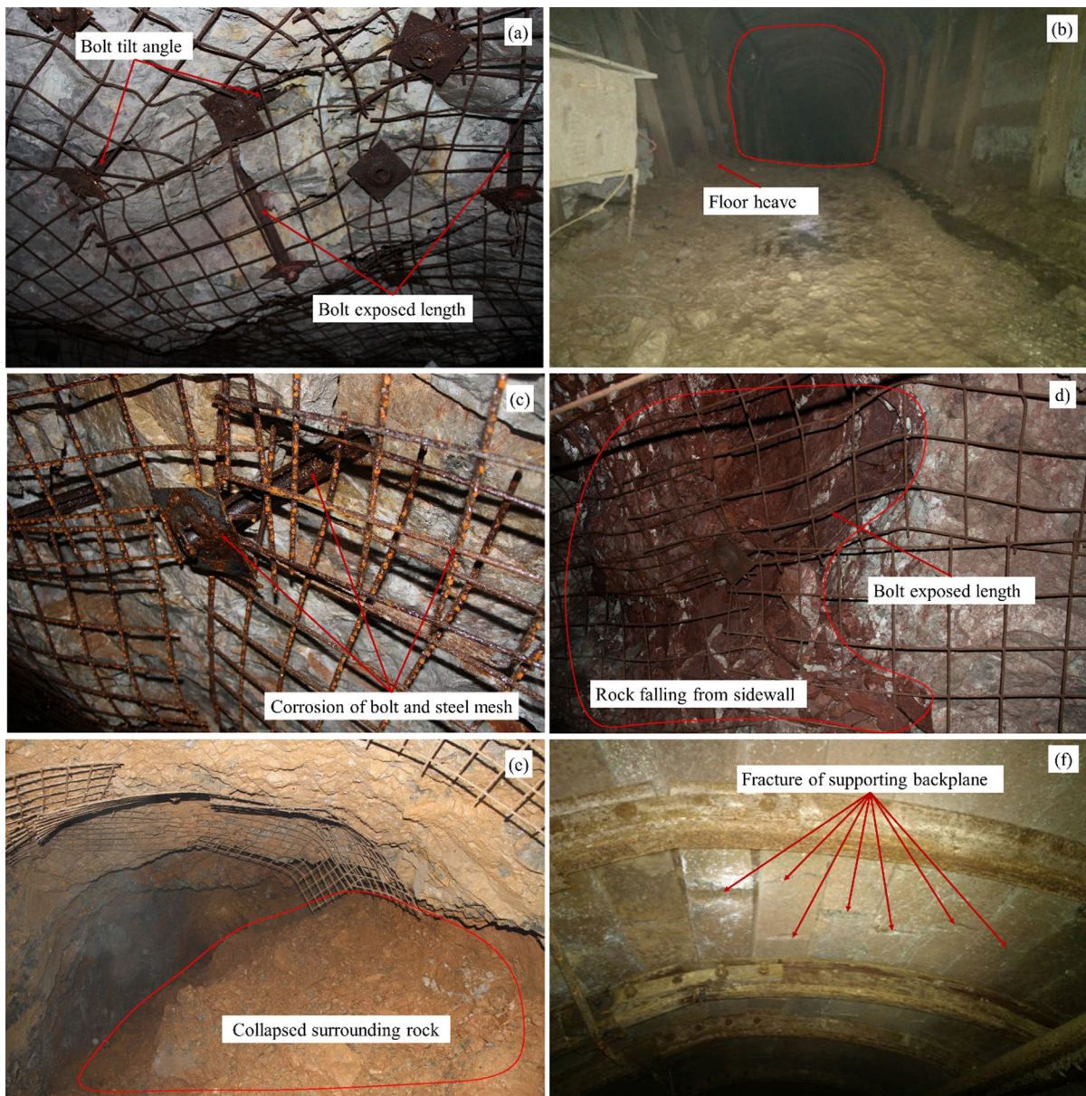
Fig. 2 Present situation and failure modes of the roadway support
