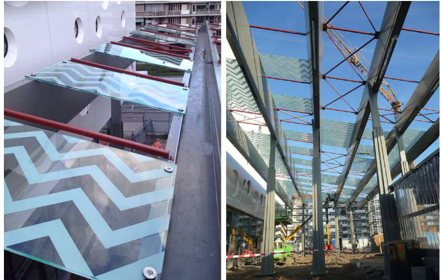
Fig. 13 The glass elements are point-fixed. Before glass installation, temporary braces were added to ensure lateral beam support
