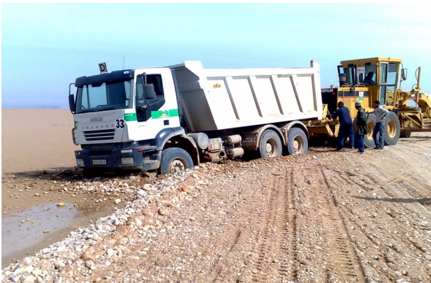
Fig. 3 Low bearing capacity of the saturated sabkha soil without geotextile
