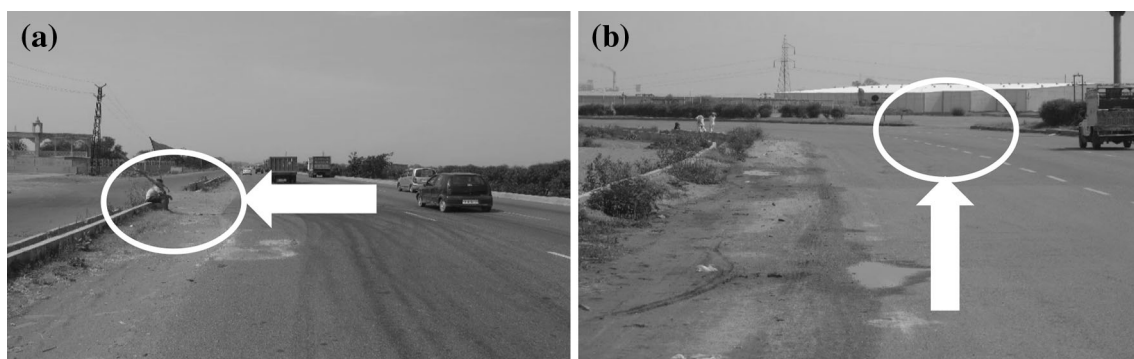
Fig. 4 a, b Typical examples of design and operation anomalies commonly observed on Indian highways
