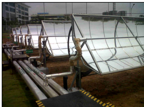
Fig. 9 Solar Parabolic Troughs (PT) array
