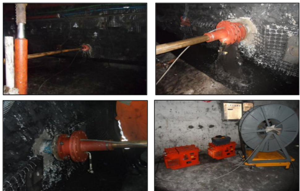
Fig. 18 Picture of CSW fracturing in situ of underground coal mine
