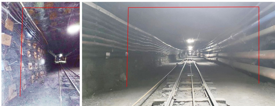
Fig. 21 Control effect of surrounding rock of roadway on site
