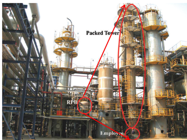
Fig. 4 Commercial demonstration of RPB for desulfurization (Qian et al. 2012)
