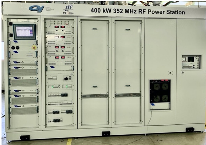
Fig. 13 One 400 kW RF power station
