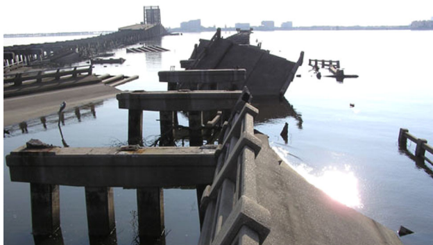
Fig. 1 Failure of the US 90 Biloxi Bay Bridge during the Hurricane Katrina (photo by Yim)
