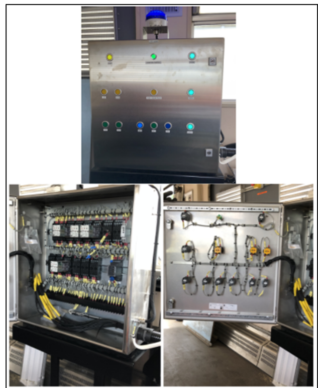
Fig. 6 Train control logic equipment, showing the exterior (above), and interior wiring (below)
