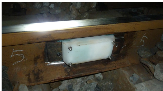
Fig. 7 Rail stress-monitoring sensor
