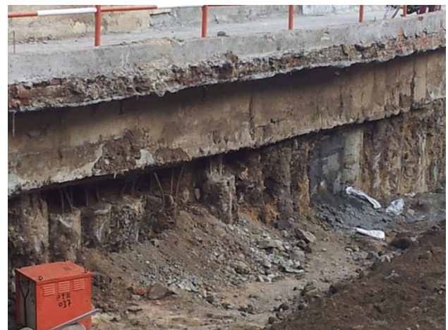
Fig. 20 Defect in shoring piles near tie beam
