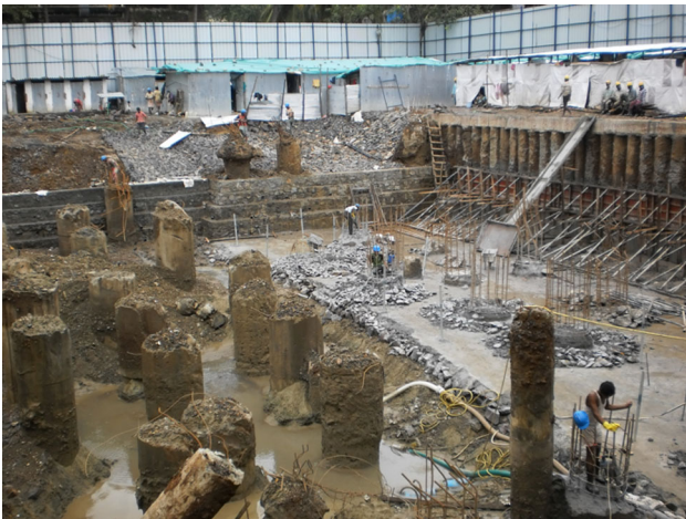
Fig. 22 Rubble wall and shoring piles without anchors for single basement in Andheri site
