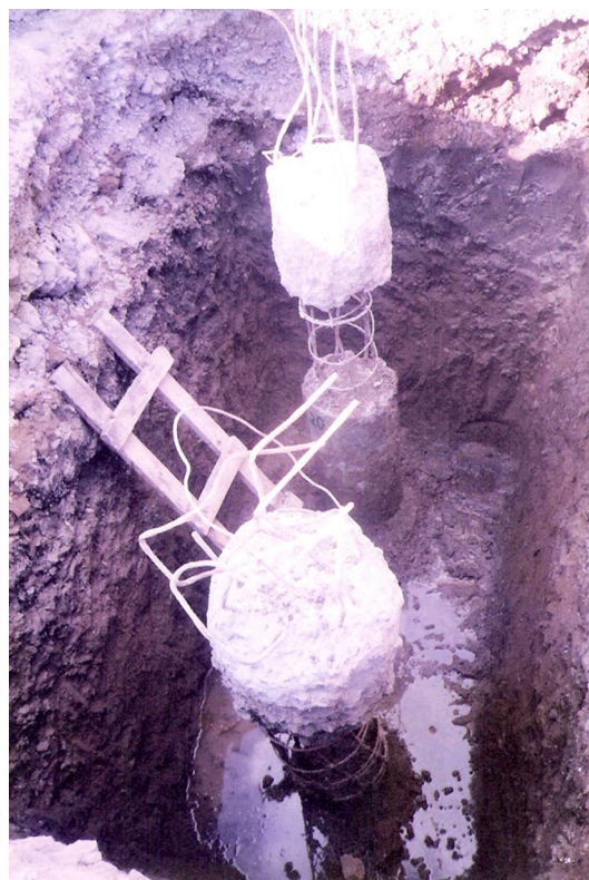
Fig. 2 Piles with severe shaft integrity problem with loss of concrete in pile shafts
