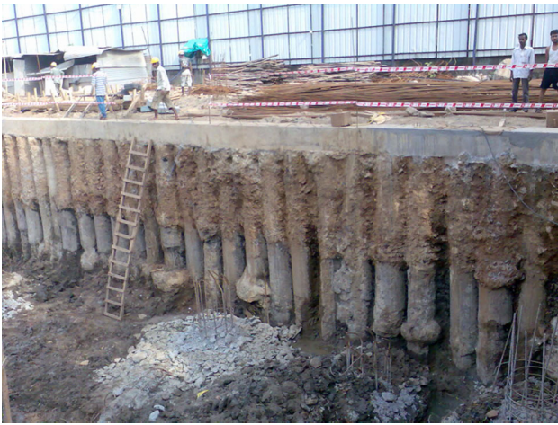
Fig. 21 Defects at tips of shoring piles
