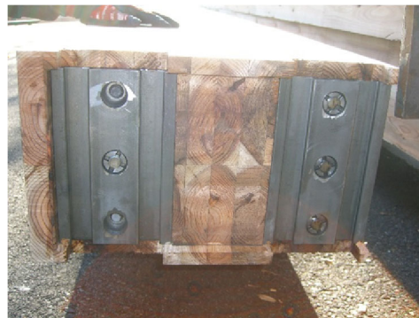
(a) Partial tensile failure of connection between LSB and plate in beam
