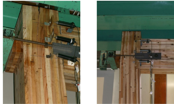
(a) Spilt at the top column (b) Bending crack on the column
