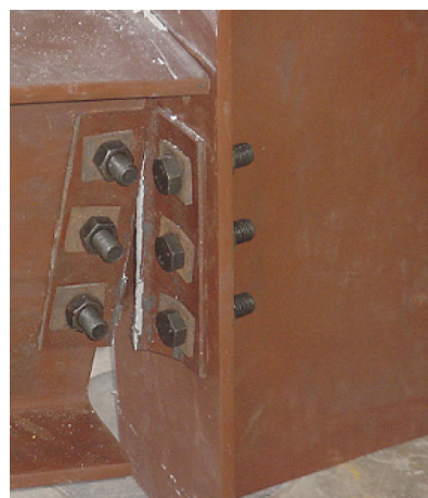
b Failure by yielding and tearing of web angle
