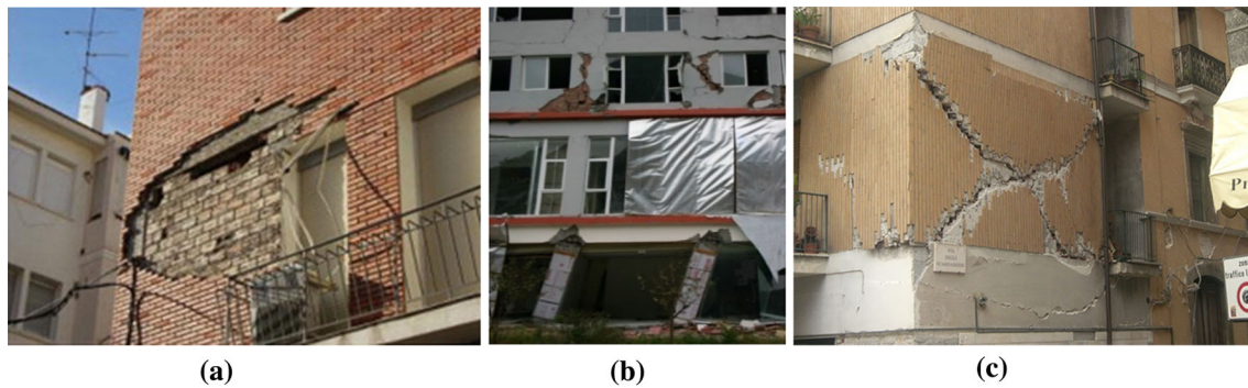
Fig. 1 a Infill walls collapse (Romão et al. 2013), b soft-storey mechanism (Costa et al. 2010) and c out-of-plane and in-plane damage mechanisms in exterior masonry walls (Romão et al. 2013)
