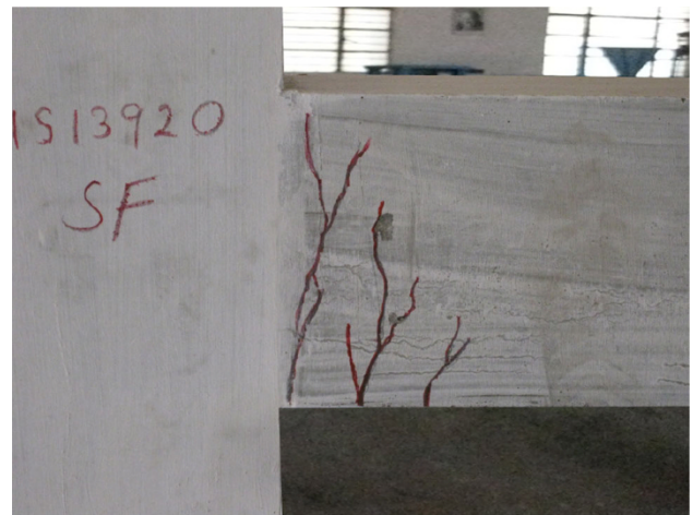
Fig. 12 Crack pattern of IS 13920 with SF
