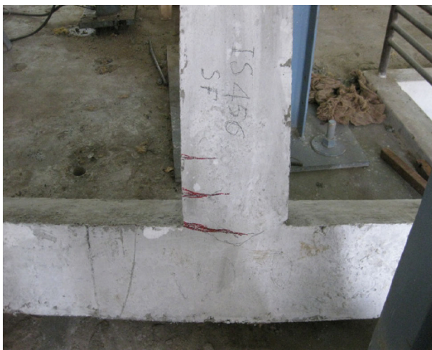
Fig. 10 Crack pattern of IS 456 with SF
