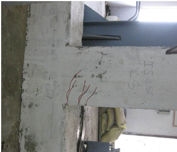
Fig. 9 Crack pattern of IS 456 CS
