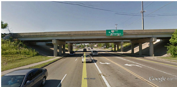
Fig. 3 South look of the study bridge (Google Earth image reproduced under “Fair Use” condition)
