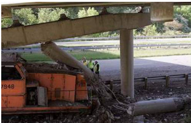
Fig. 1 Detached cap from girders due to a railroad locomotive collision on I-74 at I-275 intersection in Cincinnati, OH
