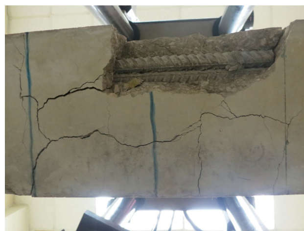
Fig. 12 Close view of the crack pattern and mode of failure associated with the bond beam (SCC-B-B2).
