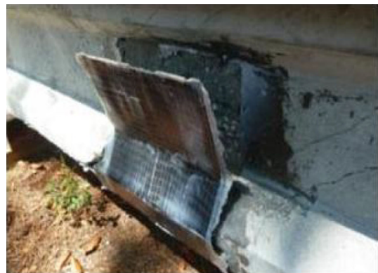
Fig. 20 Debonding of CFRP U-wrapping.
