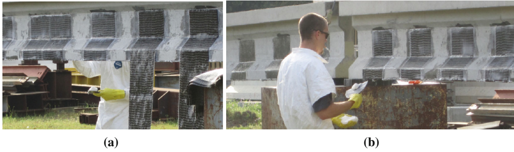
Fig. 4 Wet layup application of CFRP fabric laminates on PS girder. a Wet layup application of CFRP. b Applying epoxy to CFRP.
