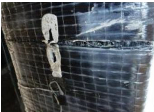
Fig. 19 Rupture of longitudinal CFRP.
