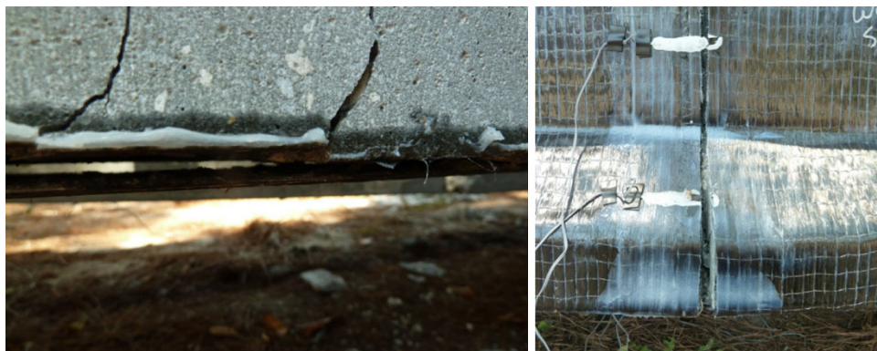
Fig. 28 (left) Debonding of soffit CFRP; (right) rupture of longitudinal and transverse CFRP.
