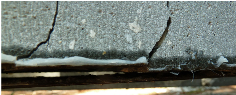
Fig. 18 Close-up of laminate debonding initiated by flexural crack development.
