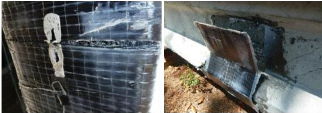
Fig. 27 (left) Rupture of longitudinal CFRP; (right) debonding of CFRP U-wrapping.
