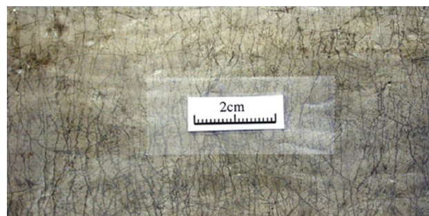
Fig. 3 Saturated crack pattern of lightweight ECC after straining to 4 % in tension.
