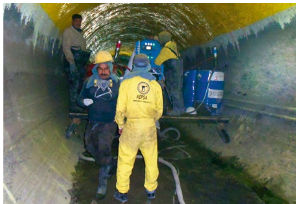
Around 110 tonnes of polyurea had been applied by the end of the project.
