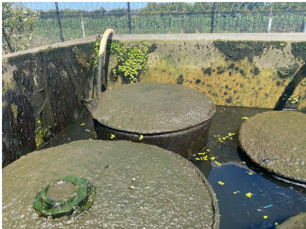
Fig. 2 The biomass growth on the filter surfaces is evident
