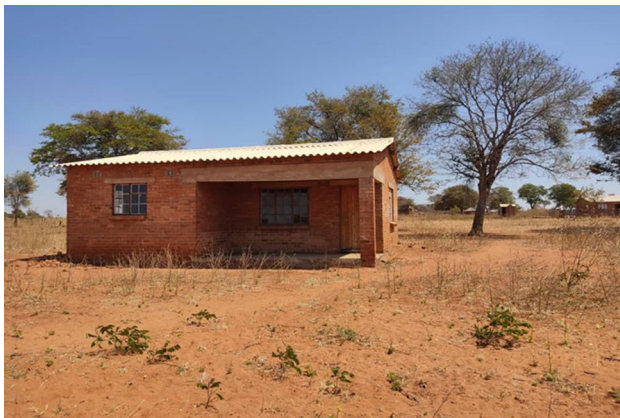
Fig. 3 Abandoned house in Sawudweni, Tsholotsho District, Zimbabwe. Photograph by N.K. Ngulube, 16 September 2022
