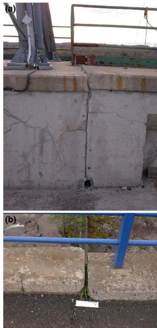
Fig. 5 Misalignment in the crest of two different concrete dams (a, b)
