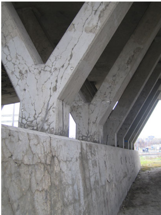
Fig. 3 Du Vallon–Charest highway interchange viaduct, in Quebec city, Canada, recently demolished because of ASR
