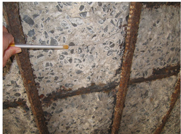
Fig. 1 Corrosion of the steel bars and spalling of the concrete in a viaduct
